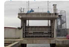
Floodgate (Other Business)
