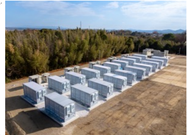
Extra-High Voltage Battery Power Plant (image: PowerX)
